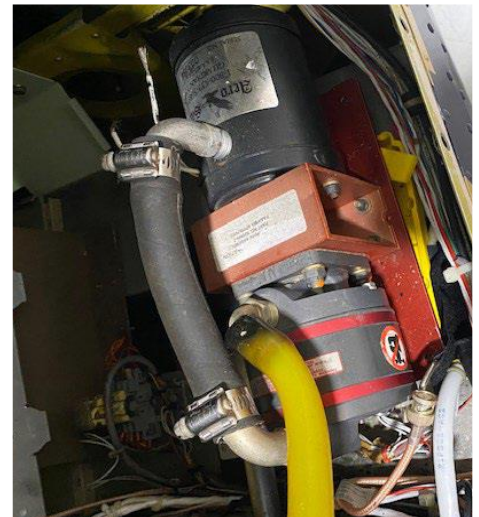
Figure 2 Standby vacuum system
