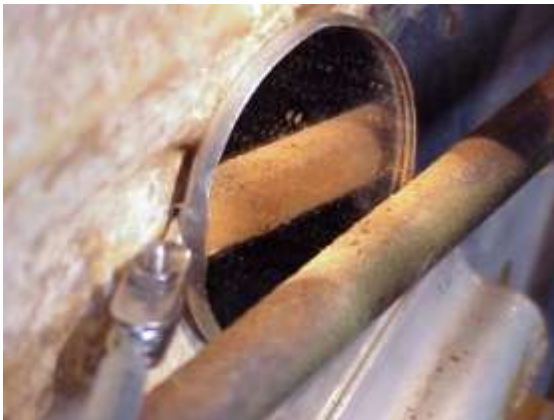
Rust on tube structure—Found during Service Bulletin inspection M20-208B
